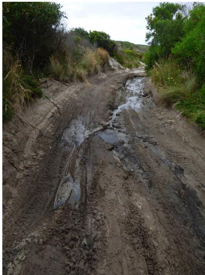
Fig.57 Damaged and eroded track to Seymour Beach
