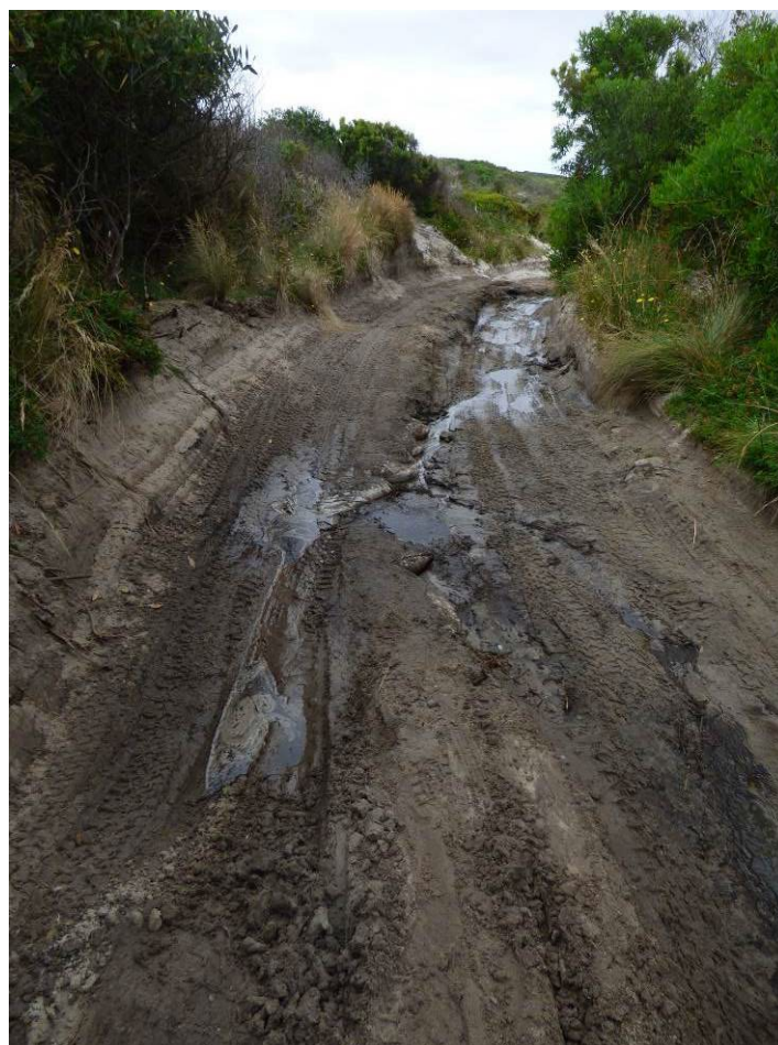
Fig.57 Damaged and eroded track to Seymour Beach
