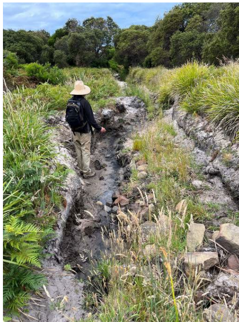
Fig. 54 Eroded track between wetland and dunes behind Templestowe beach – close this track, rehabilitate and ensure drainage does not continue to exacerbate the erosion problem.
